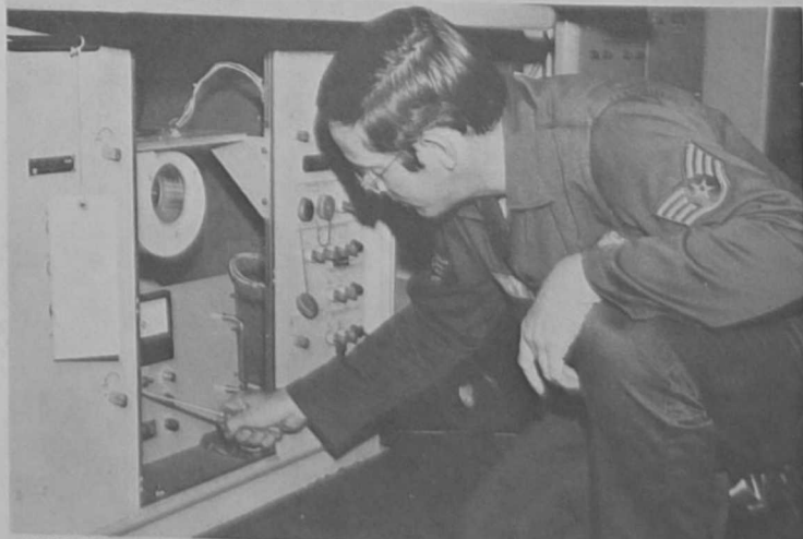
YOKOTA AB, Japan - SSgt. Louis M. Drury, a maintenance technician with the 20th Weather Squadron here makes an adjustment to the AN/FPS-77 Console Line Voltage Regulator. Sergeant Drury received a $200 suggestion award which resulted in proper procedures appearing in the technical order and assured proper equipment testing with a reduction of equipment down time. (U.S. Air Force Photo)
